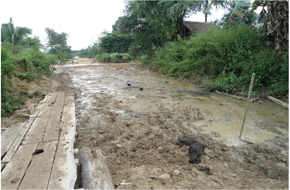
Road damaged by mining trucks
